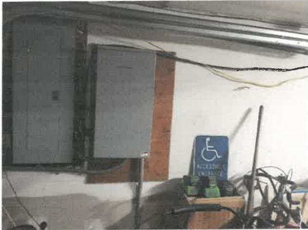
Photograph (13): Unsupported nm wires.
